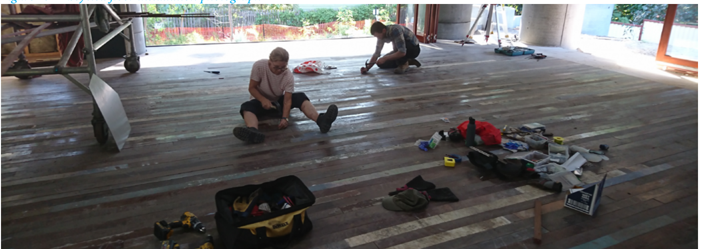
Family and friends installing Wandoo floor from Subiaco Markets. Culturally significant, and recycled
